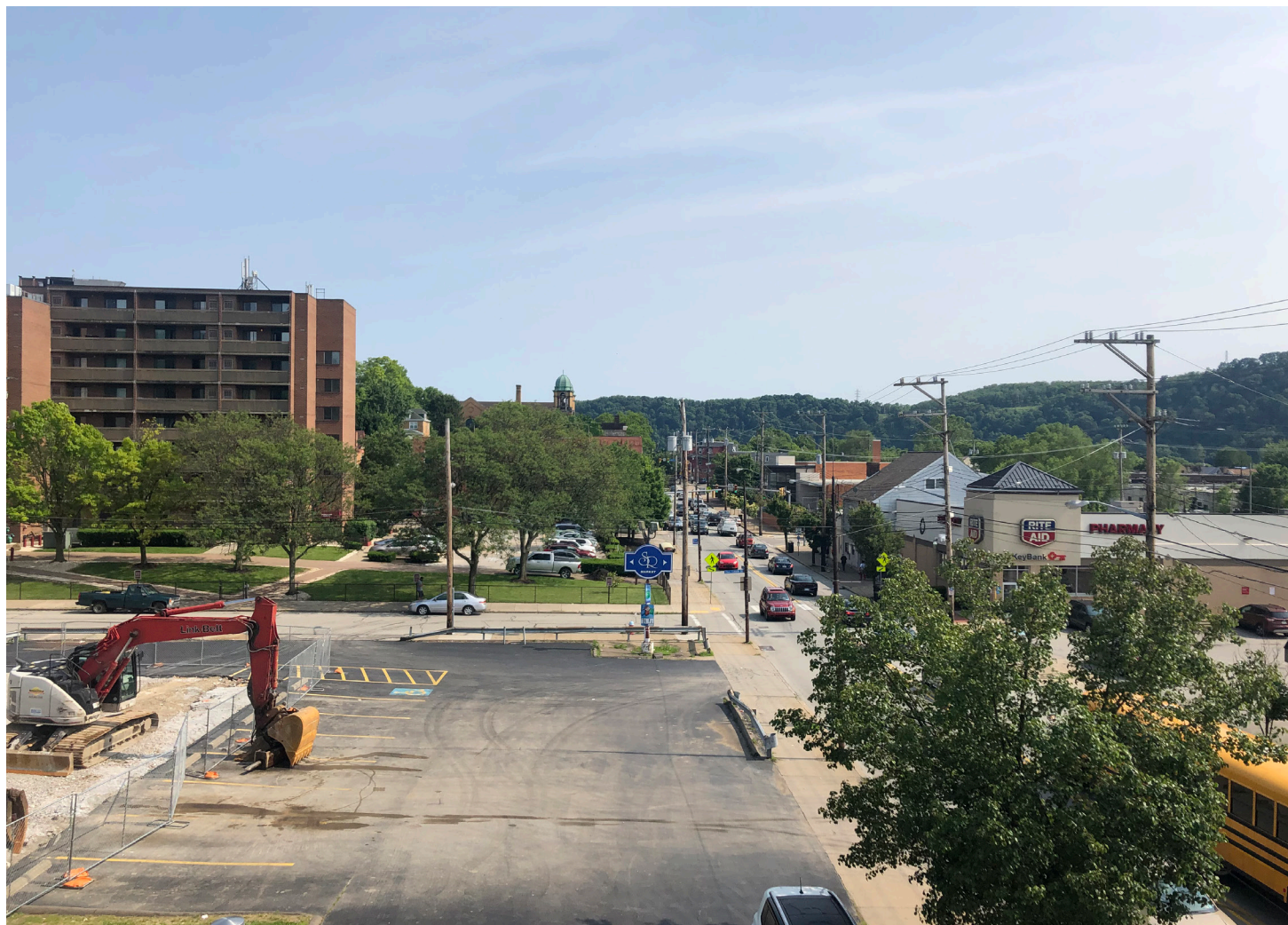
A view down Second Avenue where the S&R Market was torn down in early June. The large street-front parking lot is planned to become a street-front building.
